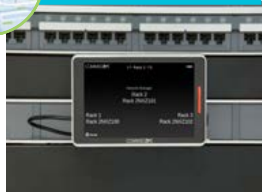
imVision manages both power and connectivity.
