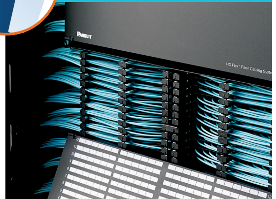
Serviceability and manageability for the next-generation data center
