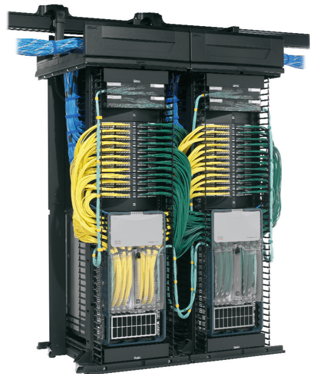
Figure 8. PANDUIT® NET-ACCESS™ Cabinet with Cisco Nexus Switch
