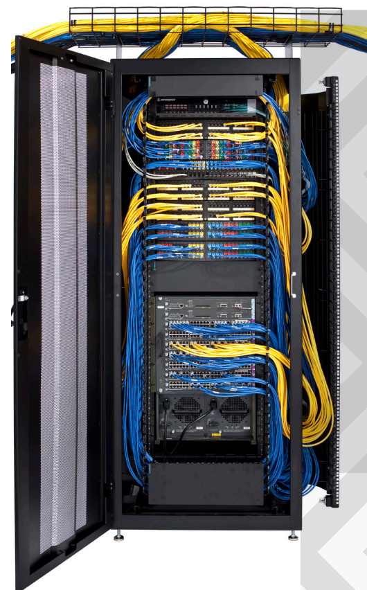
Physical support should be flexible and scalable to accommodate new equipment and have options to help manage airflow.
