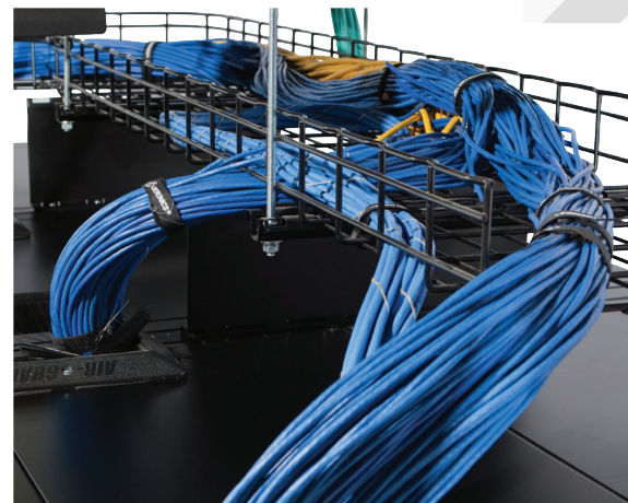
Integrated pathways reduce installation time and minimize pathway elevation changes.
