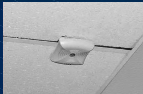
These types of openings in the ceiling tile are undesirable in a healthcare environment.
