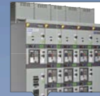
Power distribution and control
