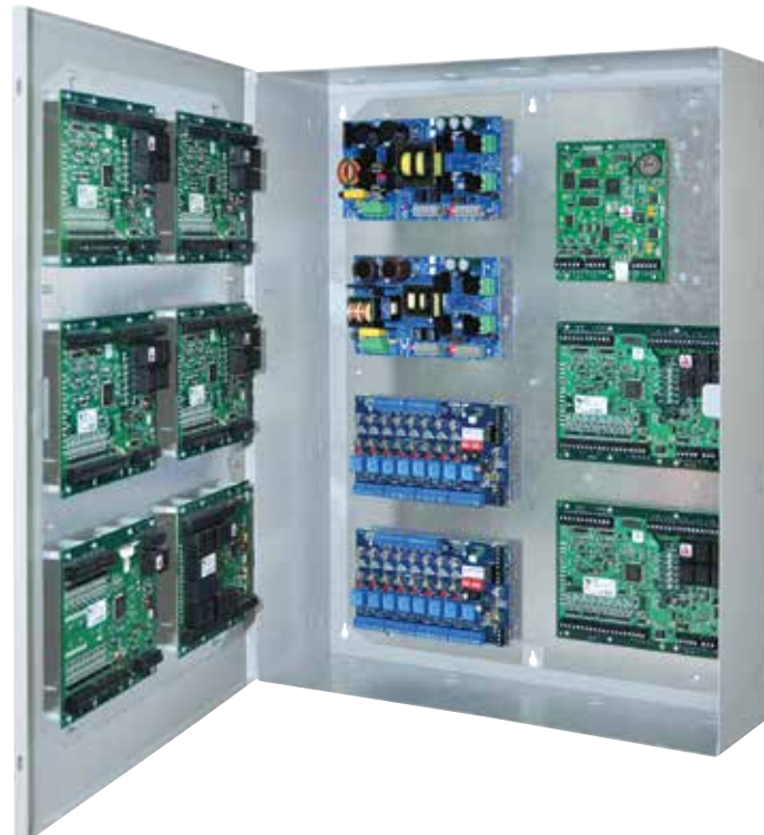
Altronix / Mercury 12-Door Access System including I/O boards with Power, utilizing TMV2 door backplane
