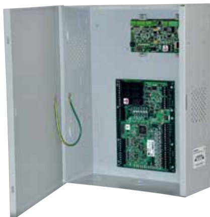
Altronix Mercury / LENEL 3-Door Access System
