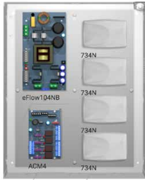
Altronix / DMP 4-Door Access System with Power
